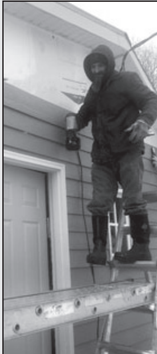
G&S Contracting employee Andy Kohl works on a remodeling job for the company.
