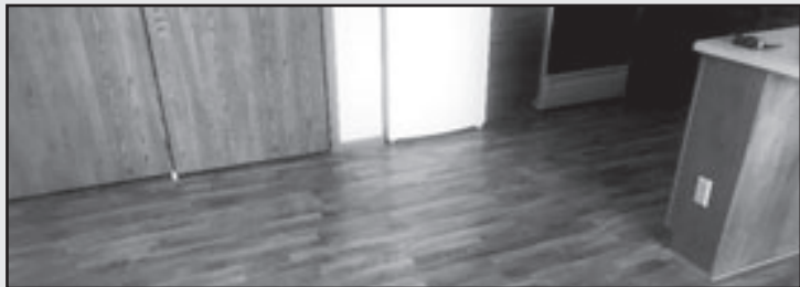
One of the remodeling projects undertaken by G&S Contracting was installing this beautiful wood floor.
